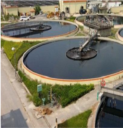
Water and sewage treatment Rain harvesting works
