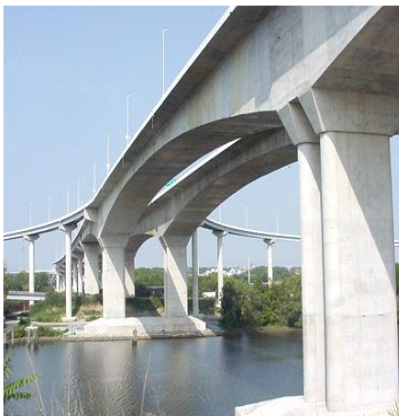
Bridges and bridge deck in aggressive environments
